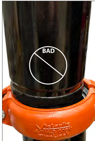
PHOTO 2 (UNACCEPTABLE) – PIPE HAS DISLODGED COUPLING
