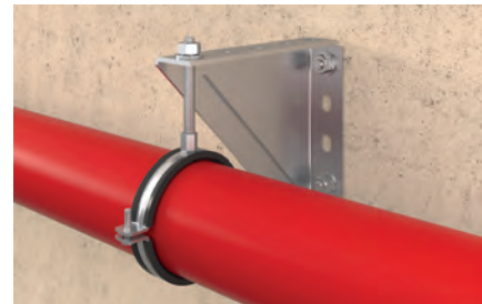
Heavy drainage pipe under angle bracket
