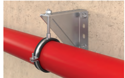
Heavy drainage pipe under angle bracket
