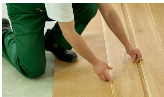
Fig. 3. The view of 3-layer wooden floorboard produced by Barlinek Inwestycje Sp. z o.o. during installation
